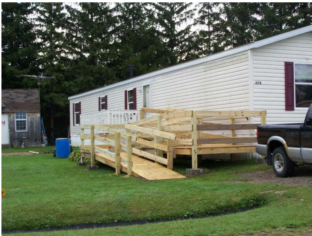
Volunteers of the United Methodist Church of Oswego constructed a ramp at the residence of Ricky Lyboul in anticipation of his sister's return home.
